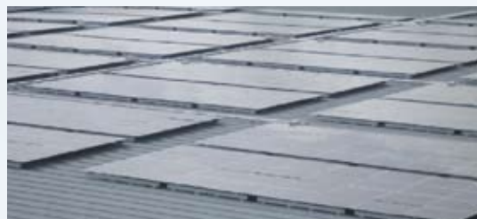
Thin-film PV cell panel installed at the new plant
