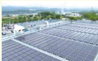
PV power generation system at the Yamanashi Plant
